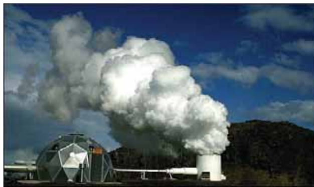
Figure 18: Geothermal Well Head and Silencer (Landsvirkjun, Iceland)
