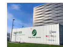
next-generation battery storage system
