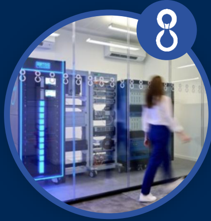
Smart Meter and Grid Lab – São Paulo
