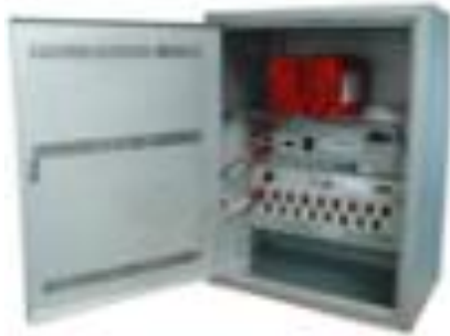
MV Remote Control Equipment
