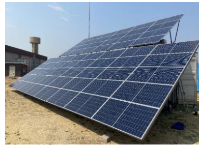
Figure 6 – 24Kw installed PV Panels
