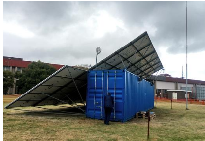
Figure 4 – 12m Containerised power plant
