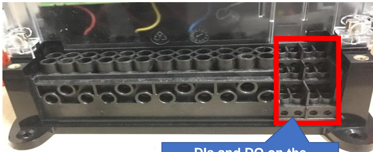
DIs and DO on the terminal block of smart meter
