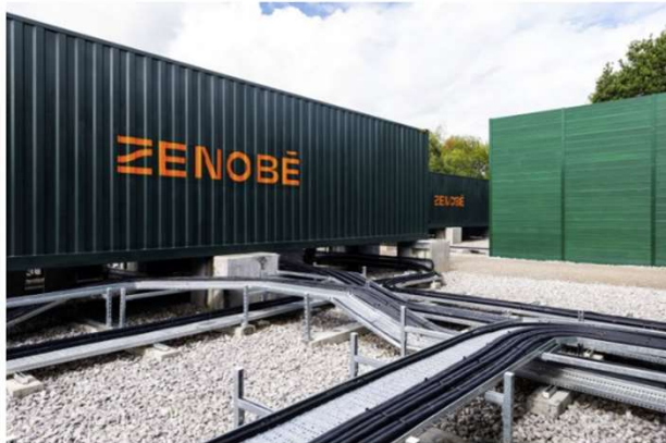
Zenobē's landmark 100MW battery storage asset at Capenhurst, Cheshire, in the UK.
