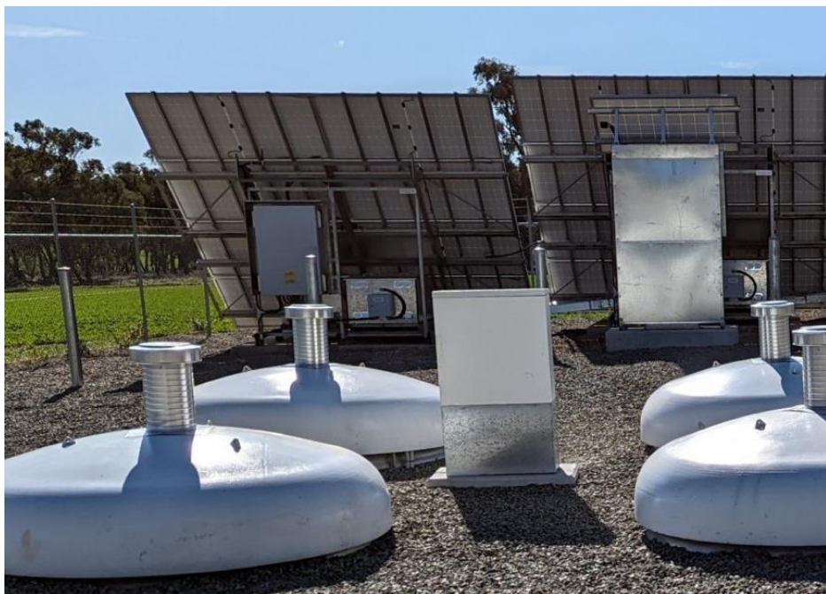
Below Grade (Australia) (4xM32 = 32kW/128kWh)
