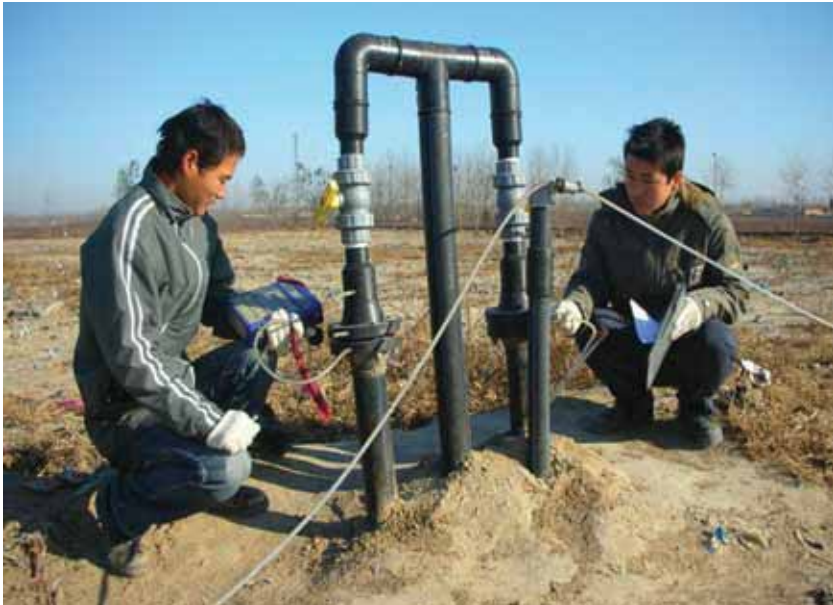
Figure 13.6 Landfill Gas Piping on Top of the Tianjin Shuangkou Landfill
