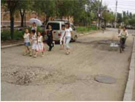
Figure 10.5 Poor Quality of a Secondary Road in Liaoning
