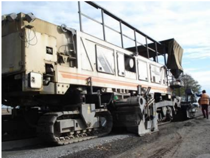
On-site recycling with bituminous emulsion and cement on Kiev/Chop road (Ukraine) (Source Egis Bceom International 2009)
