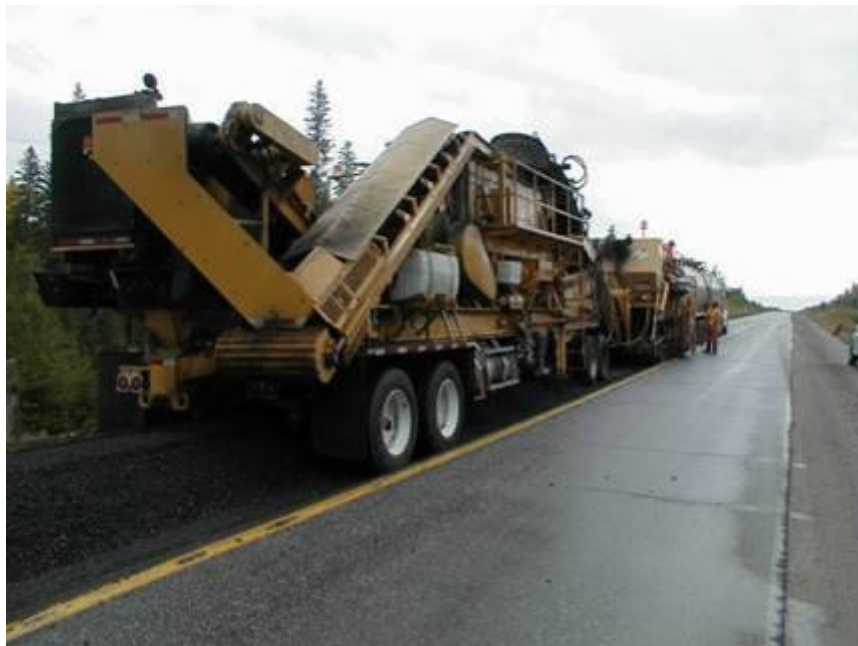
Cold In-place Recycling (CIR) construction train and equipment. (Source: Ministry of Transportation of Ontario)
