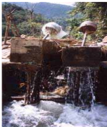
Photo 2.6: Low-head propeller turbine (Vietnam)
