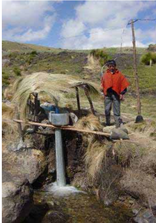
Photo 1: Picohydro Installed in Ecuador for Family Use
