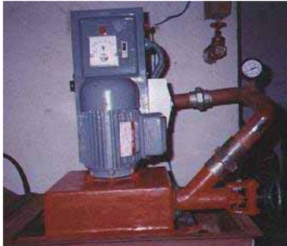
Photo 2.4: Medium-head cross-flow turbine (c/o PRRM, Philippines)
