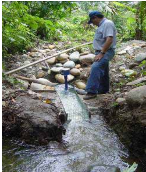
Photo 4.10: Vietnamese 200 Watt Low-Head Picohydro “Propeller” Unit Installed in Ecuador
