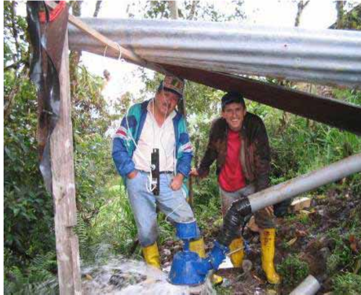
Photo 4.11: Vietnamese 200 Watt Medium-Head Picohydro “Turgo” Unit Installed in Ecuador
