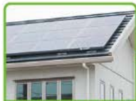
Solar panel (3.2 kW)
