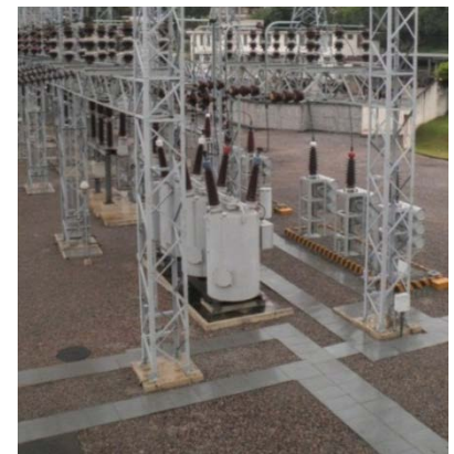
30-year old circuit breakers
