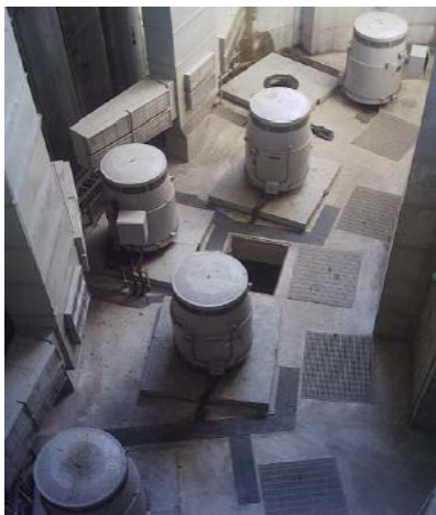
Wastewater treatment facility pumps
