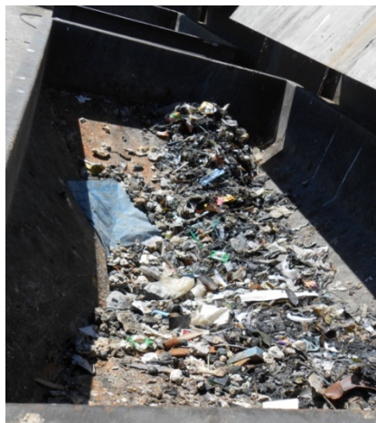
Removed trash, which reduces pump efficiency at treatment facility pumps
